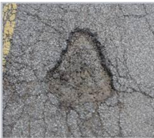
Fig 1: Examples of a pothole
